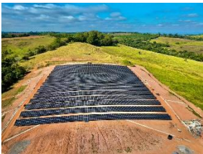
Figure 8. Overview of power plant D located in industrial area of Três Corações city, Minas Gerais state, Brazil.
