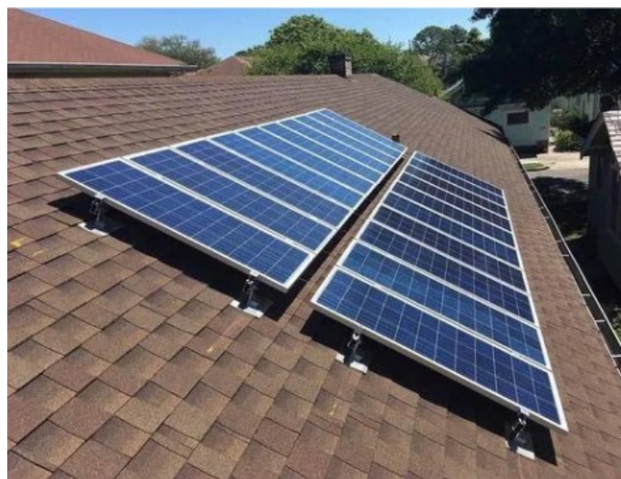
Figure 7: 6 kW solar system on a rooftop
